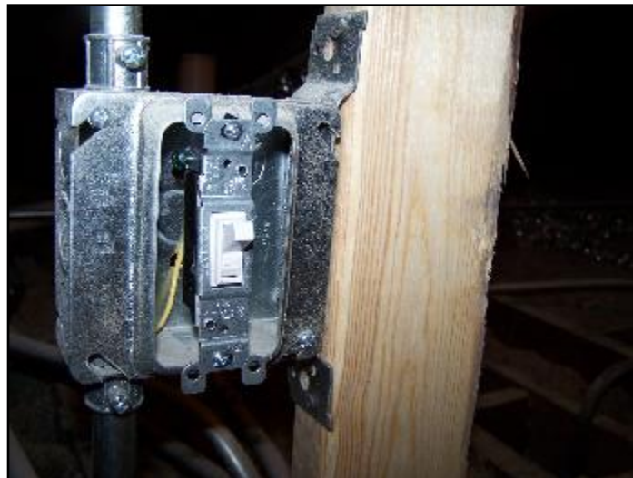
Missing switchplate cover
