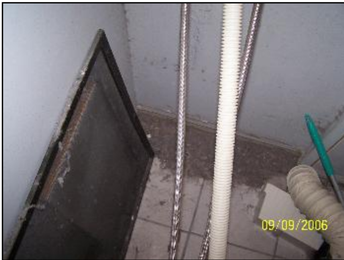
Lint pile behind dryer. Fire Hazard.
