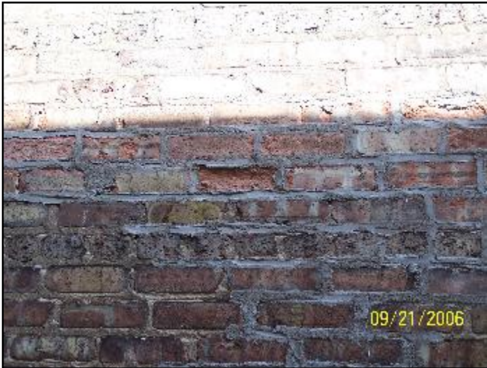
Spalling, masonry deterioration
