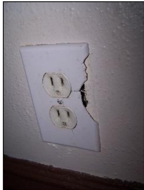
Cracked cover, paint clogged - replace
