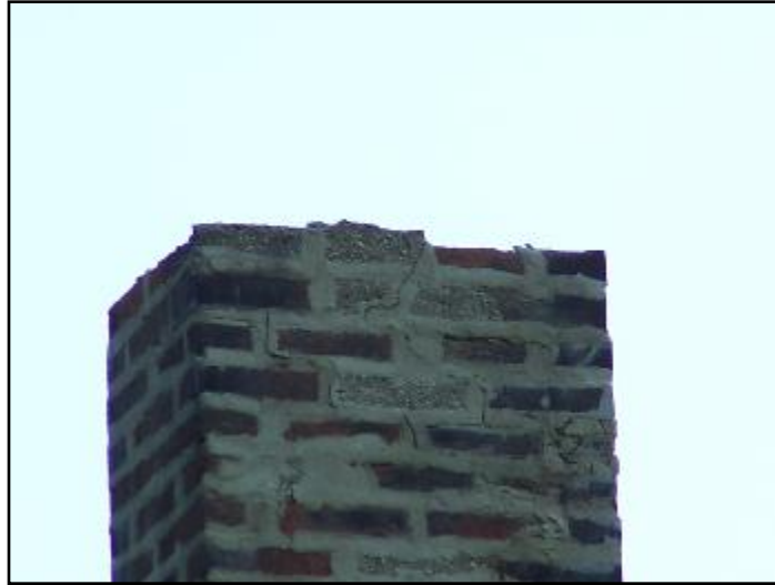
Missing chimney cap; previous repairs
