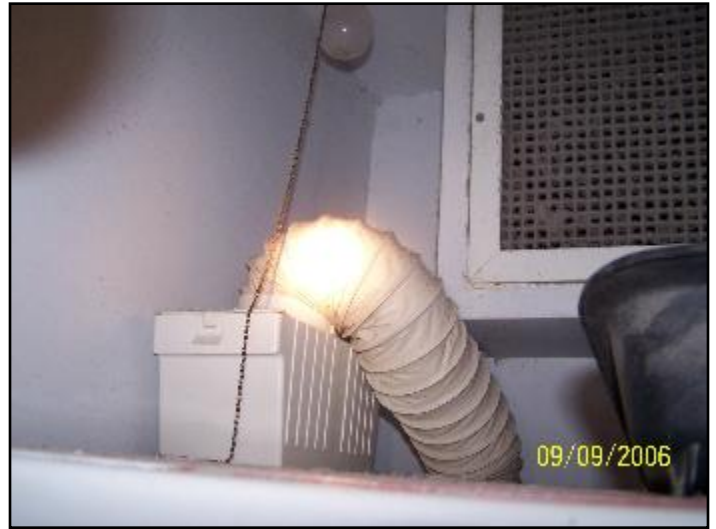
Lint trap, vinyl hose are fire hazards.
