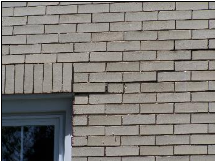
Masonry crack at window edge
