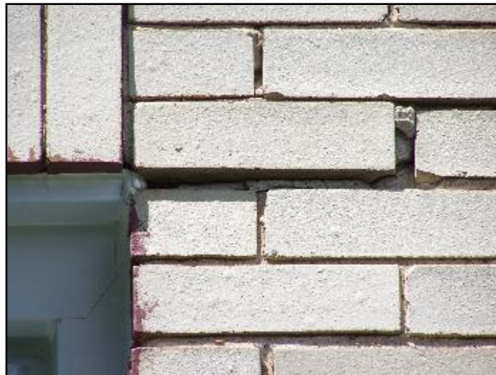
mortar damage from rusting lintel
