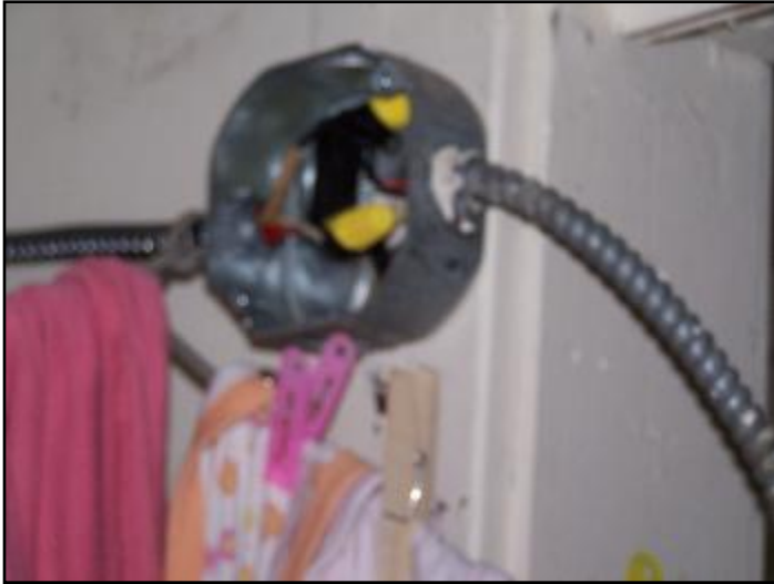
Open junction box
