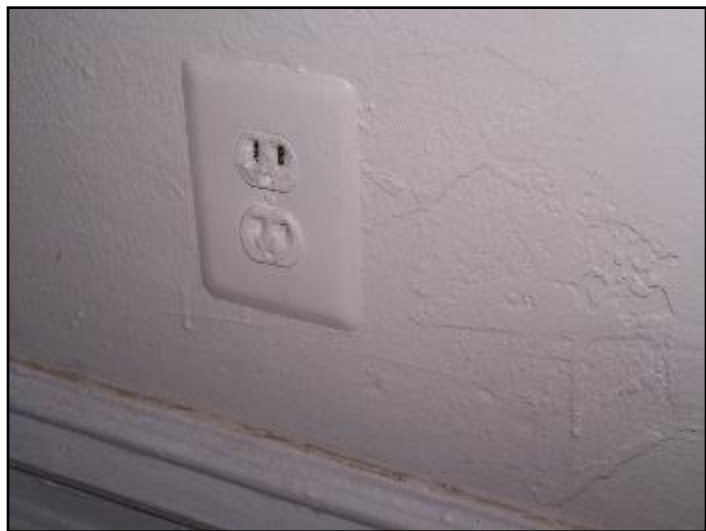
Paint damaged - replace
