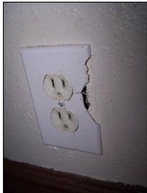
Cracked cover, paint clogged - replace
