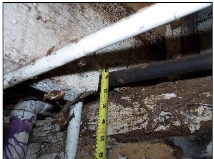
Joist notched too deep
