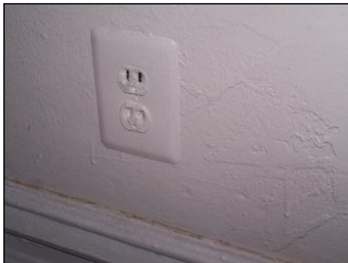
Paint damaged - replace
