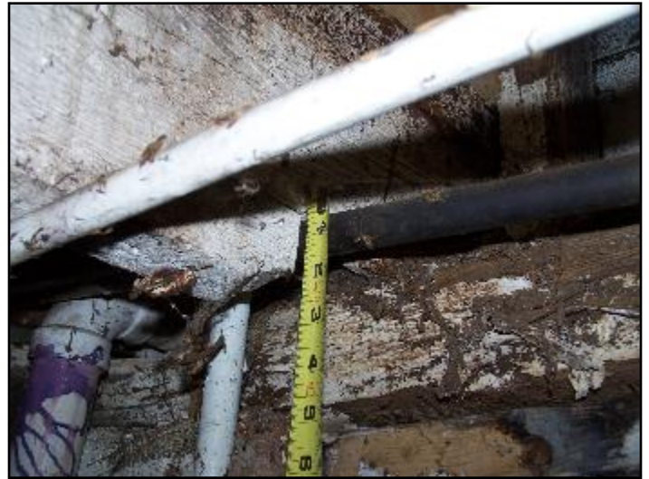
Joist notched too deep
