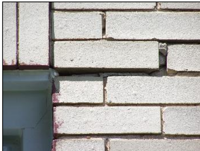
mortar damage from rusting lintel
