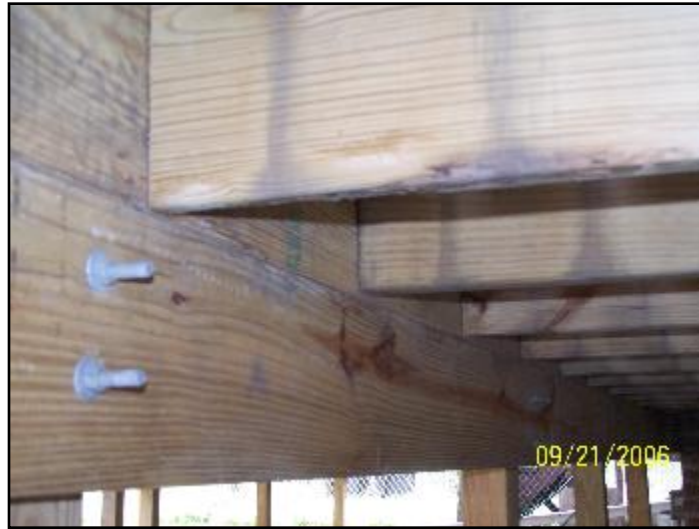
Joist Hangers Missing. Inadequate support.
