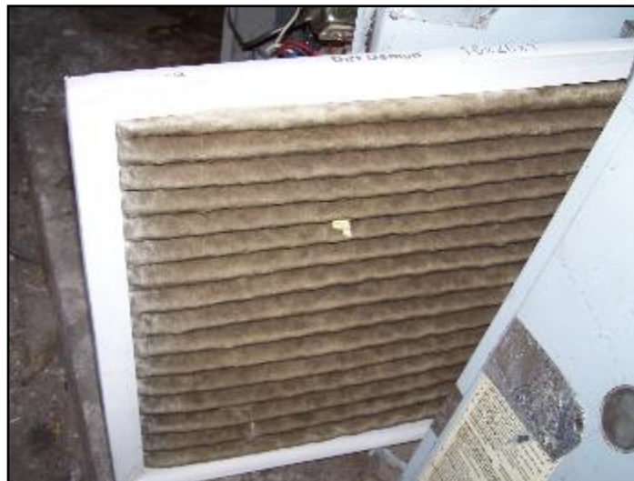
Replace dirty furnace filters
