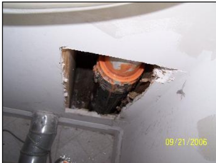
Leaking waste stack
