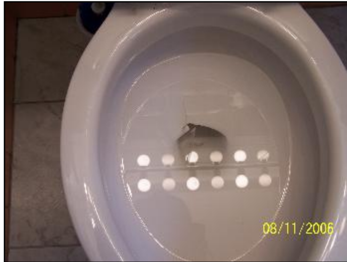
Cracked toilet bowl
