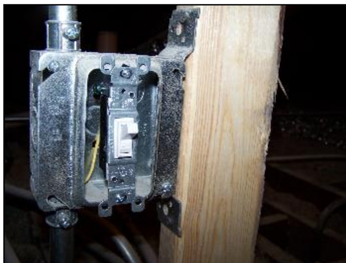
Missing switchplate cover
