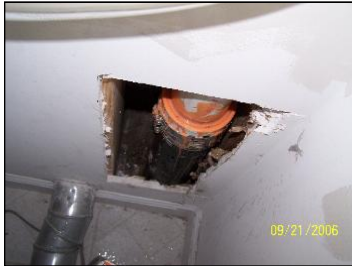
Leaking waste stack
