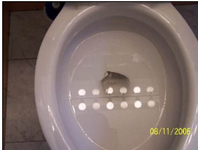
Cracked toilet bowl
