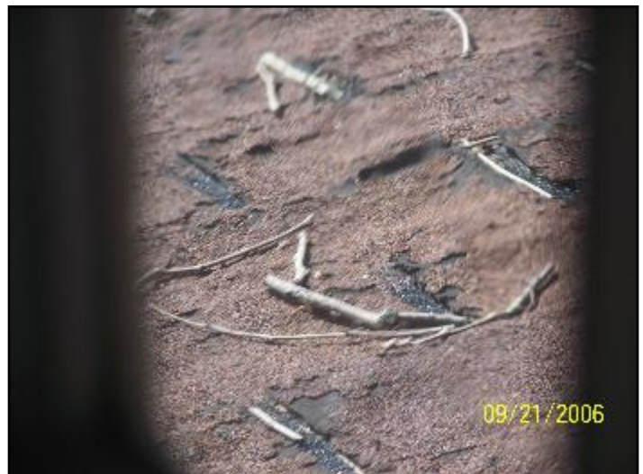
granule loss, surface deterioration
