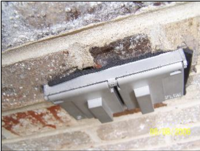
Exterior outlet not watertight, needs GFI
