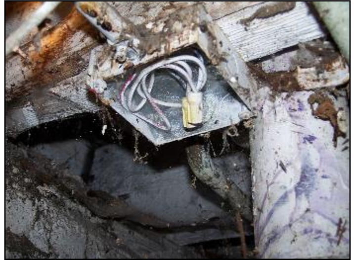
Open junction box
