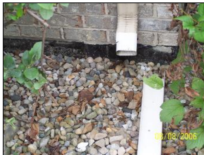
Downspout too close to house
