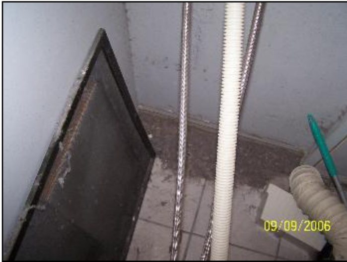
Lint pile behind dryer. Fire Hazard.
