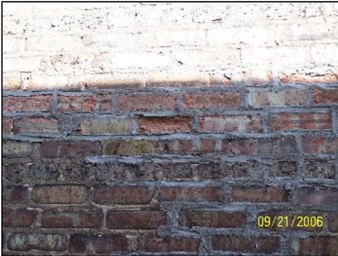
Spalling, masonry deterioration
