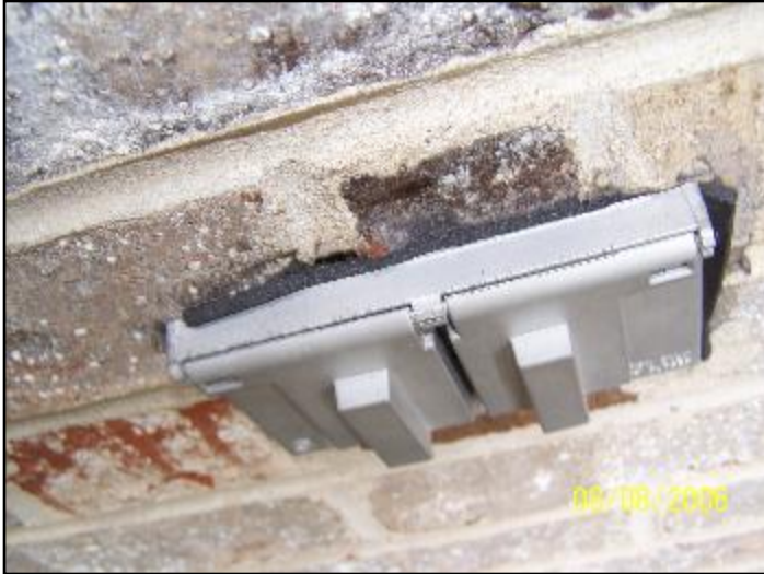
Exterior outlet not watertight, needs GFI
