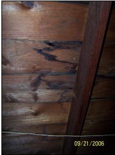
water stains on duckboards
