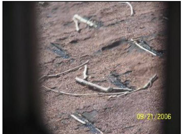
granule loss, surface deterioration
