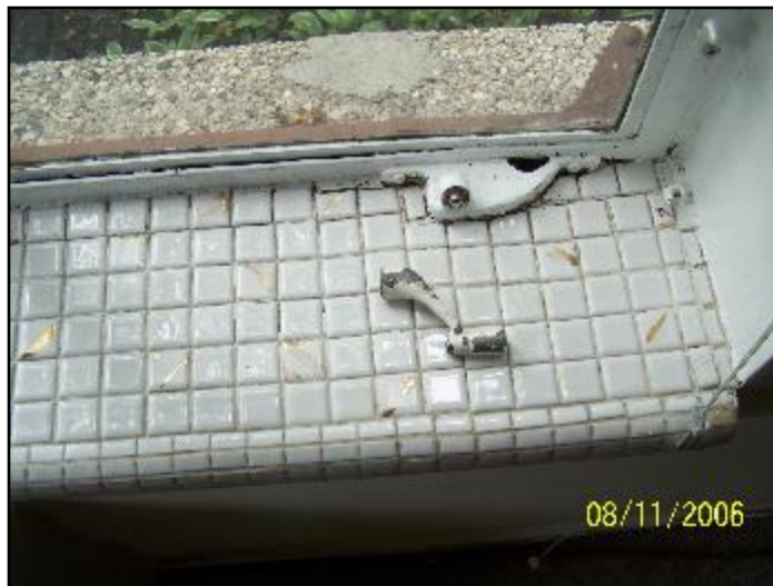
Broken window hardware
