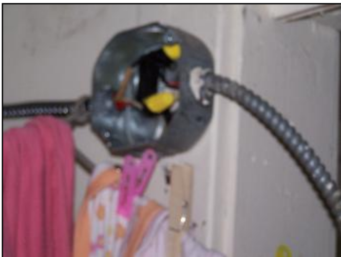
Open junction box
