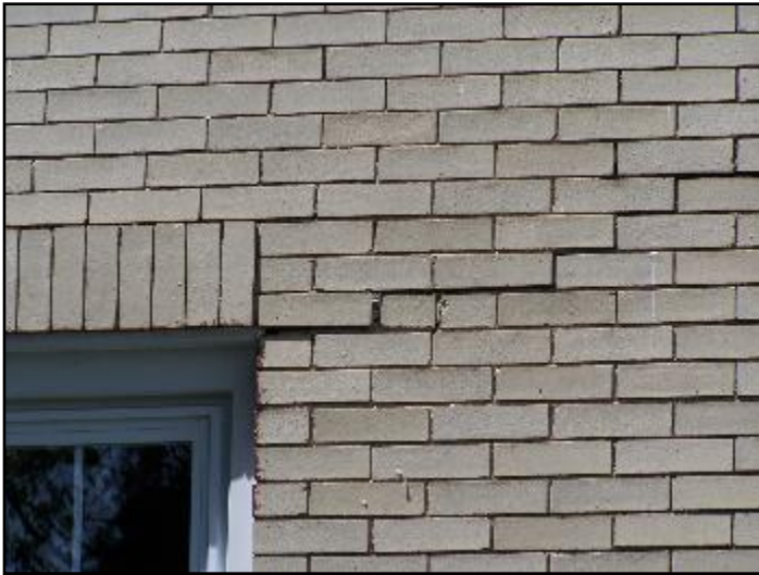
Masonry crack at window edge
