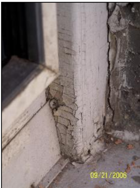
Scraping, painting, caulk needed throughout
