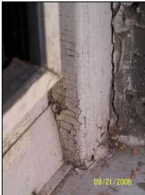
Scraping, painting, caulk needed throughout
