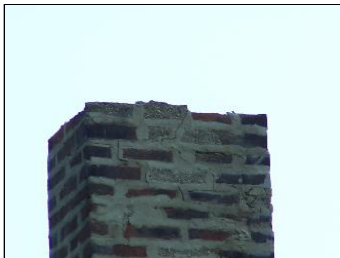
Missing chimney cap; previous repairs
