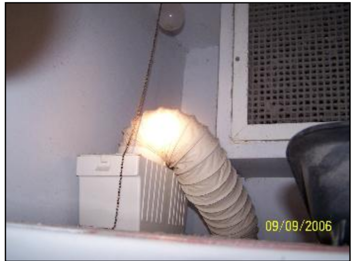
Lint trap, vinyl hose are fire hazards.
