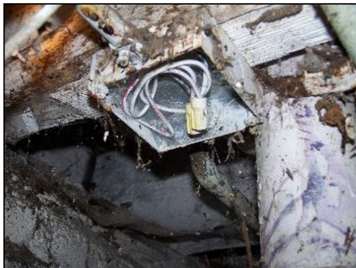
Open junction box
