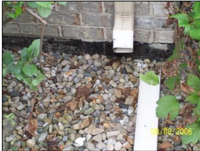
Downspout too close to house
